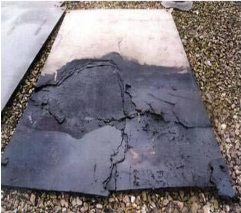
Figure 1: Flashover failure along barrier board
